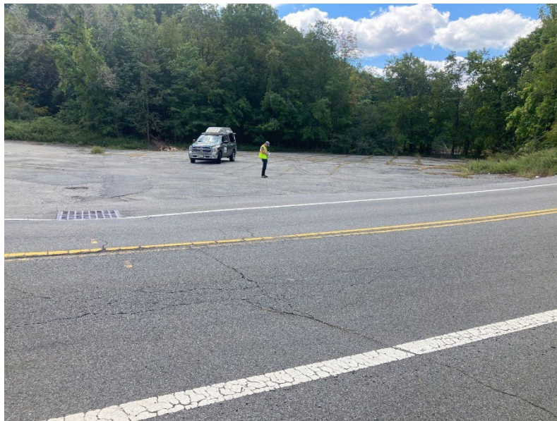
Photo 29: Mount Hope Road roadside inlet and part of surrounding parking lot area
