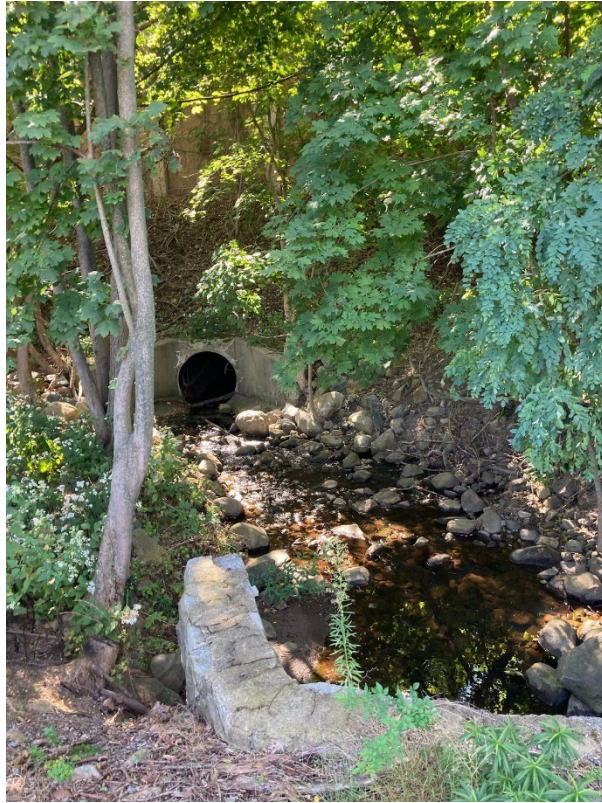
Photo 43: Outlet of street drainage system that drains to piping system under Route 80
